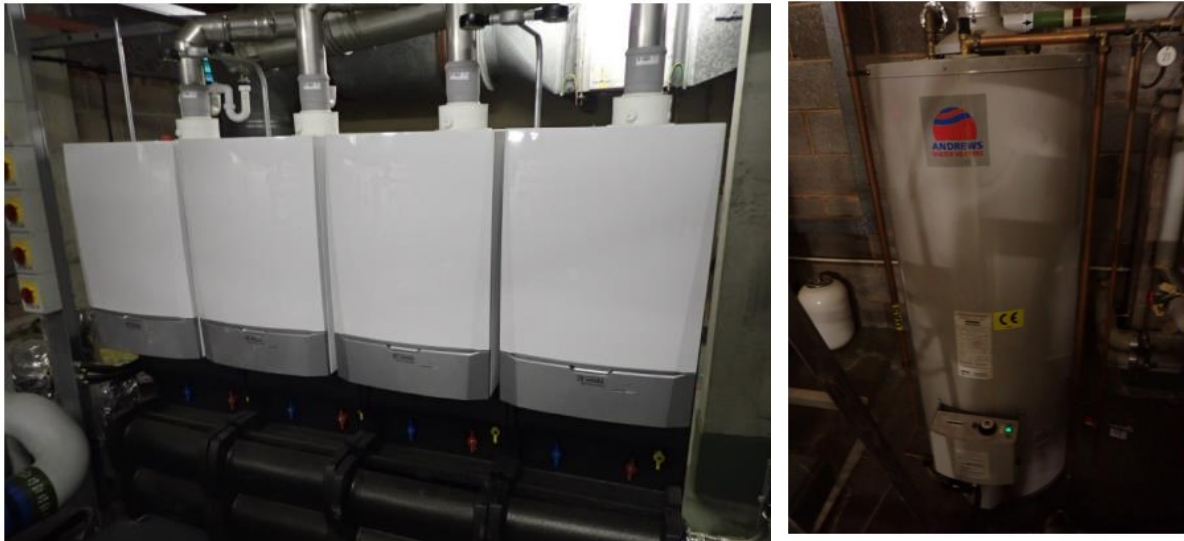
Figure 5 and 6: The current gas-fired boilers and hot water heater used in the building.
