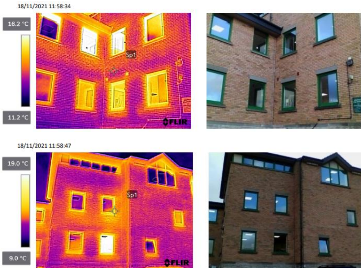
Figure 7 and 8: Outputs from the thermal imaging survey suggesting some of existing PIR board insulation in the walls could be performing poorly around windows.
