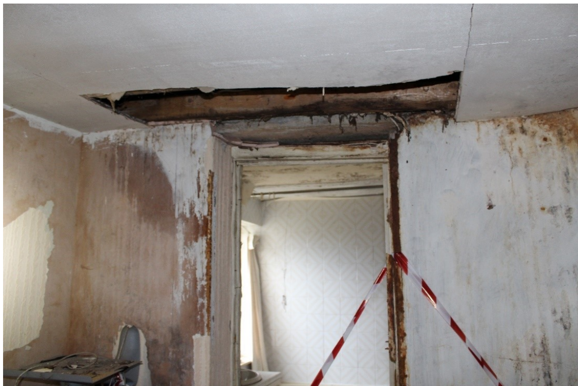
Fig. 9 Roof leaks have caused decay, collapsed and loss of the historic structure below in multiple areas over 3 floors.
