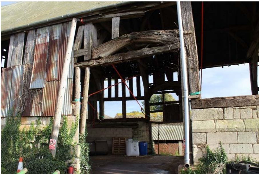
Fig.9 Entrance is in a precarious condition and still used by heavy farm machinery.
