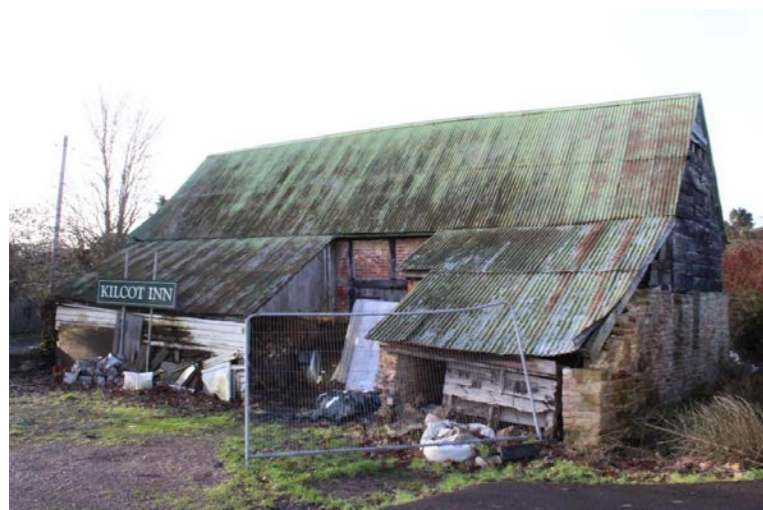
Fig. 3 Front and side elevation - in poor condition
