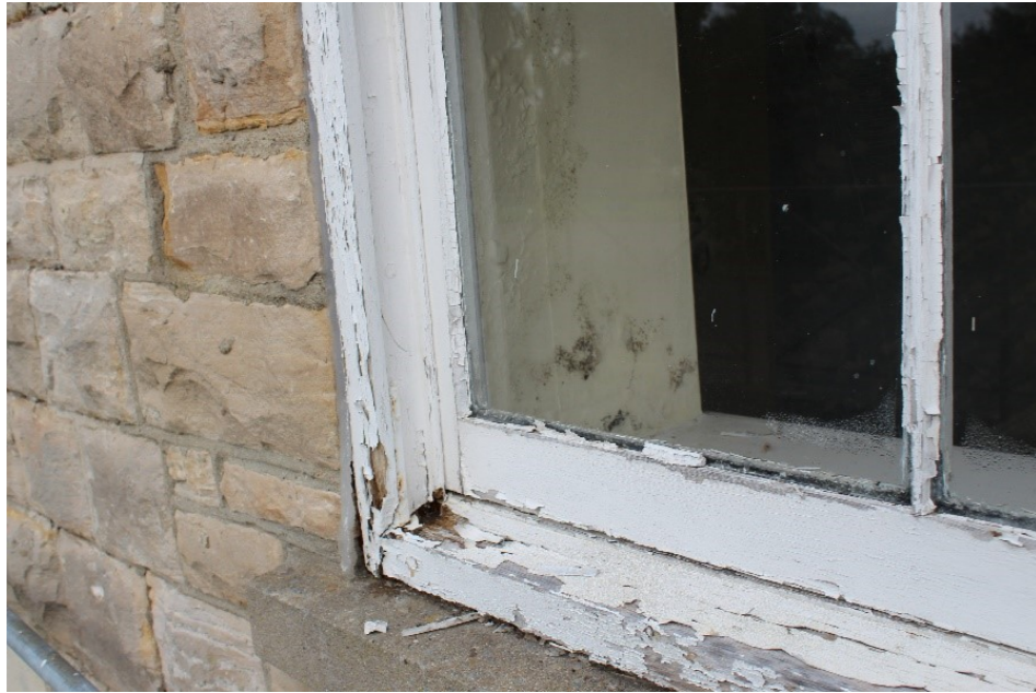
Fig. 13 Defective timber windows
