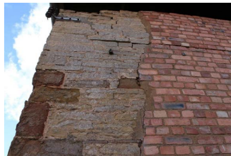
Fig. 8 Cracking evident in between modern infill brick and original stone
