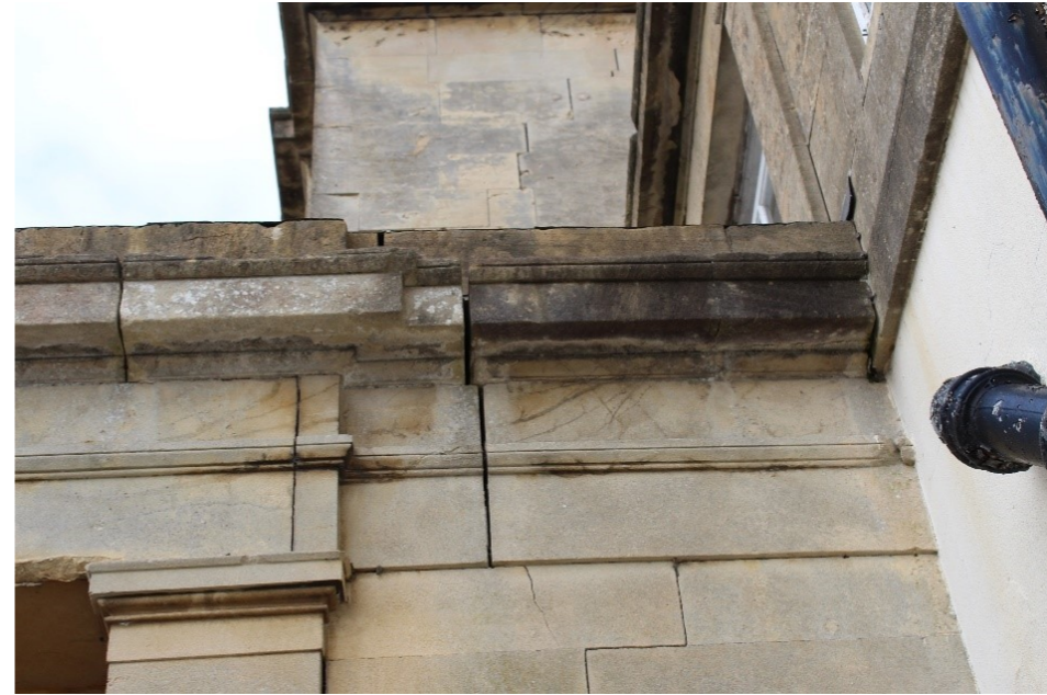
Fig. 6 Side of colonnade - cracking evident in stonework
