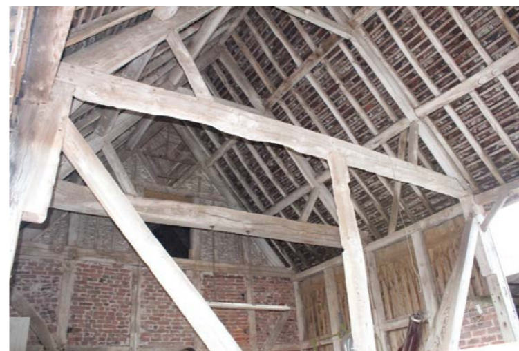
Fig. 8 Internal view of roof and internal timber framed wall infilled with wattle and daub and brick infill panels below
