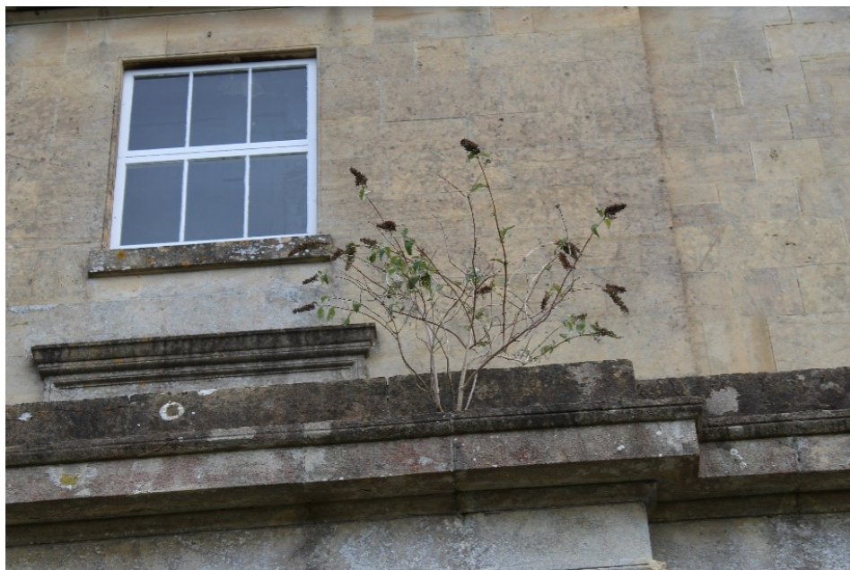
Fig. 17 Vegetation growing in wall - side elevation
