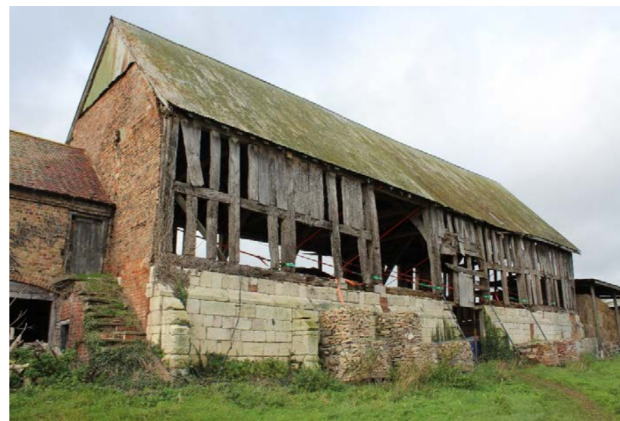
Fig. 2 Side and rear elevation of deteriorated barn.
