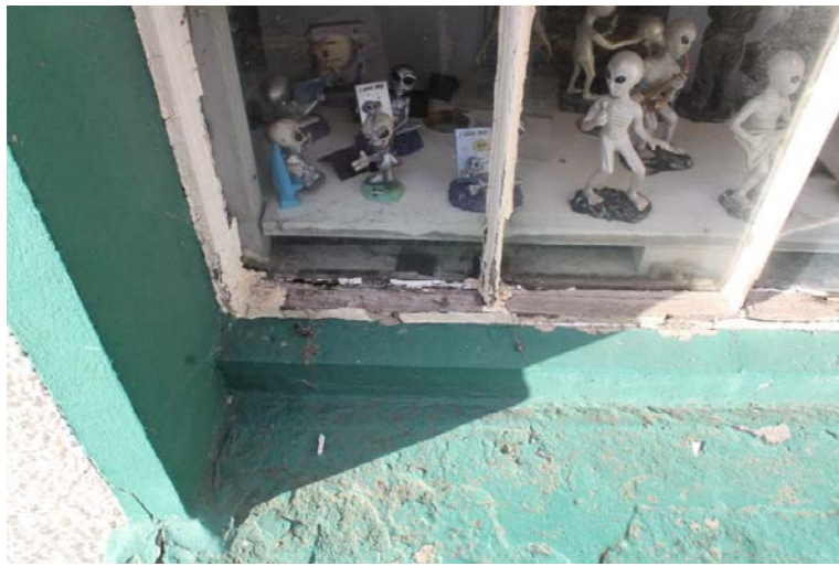
Fig. 3 Front left ground floor timber window frame - in poor condition
