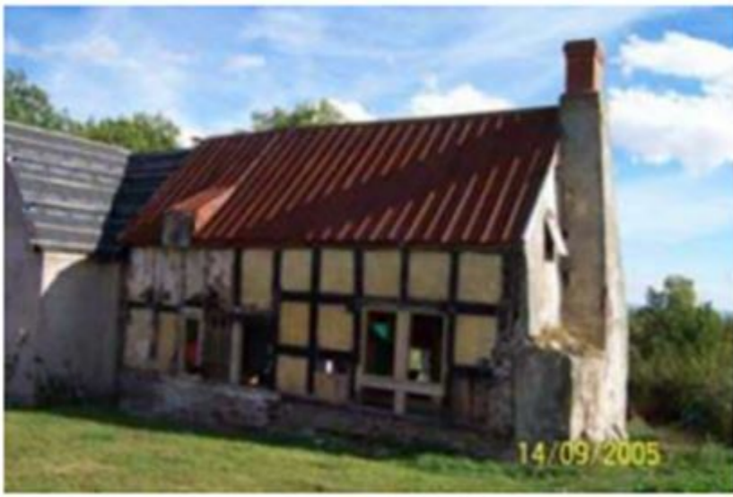
Photo taken in 2005. Front elevation and steel roof sheets protecting the roof.
