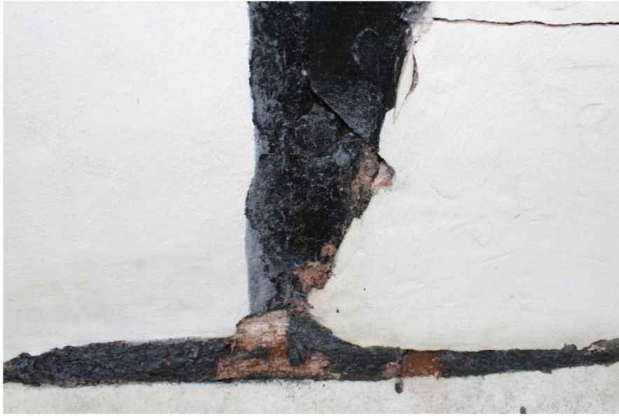
Fig.7 Trapped moisture is causing harmful decay of the original external timber frame
