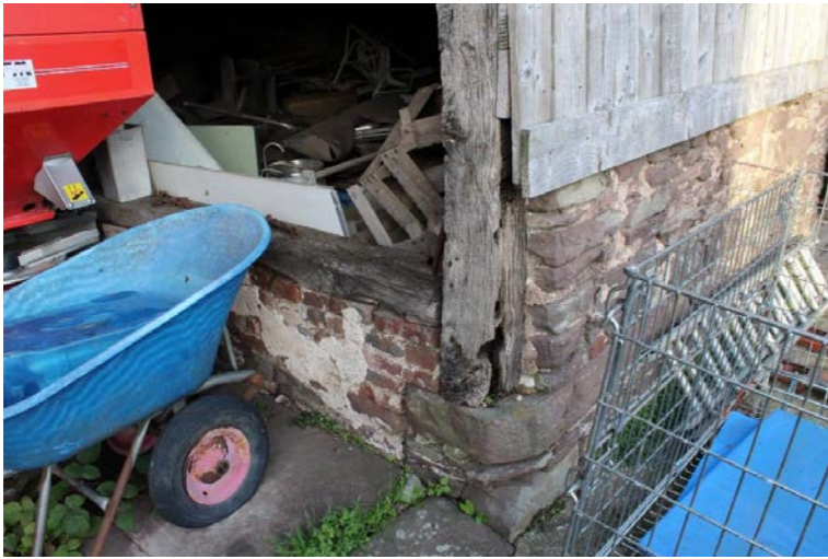
Fig. 5 Defective door frame to side elevation opening 1
