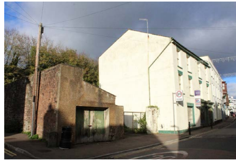
Fig. 4 Side elevation - detached curtilage garage in foreground - is in poor condition
