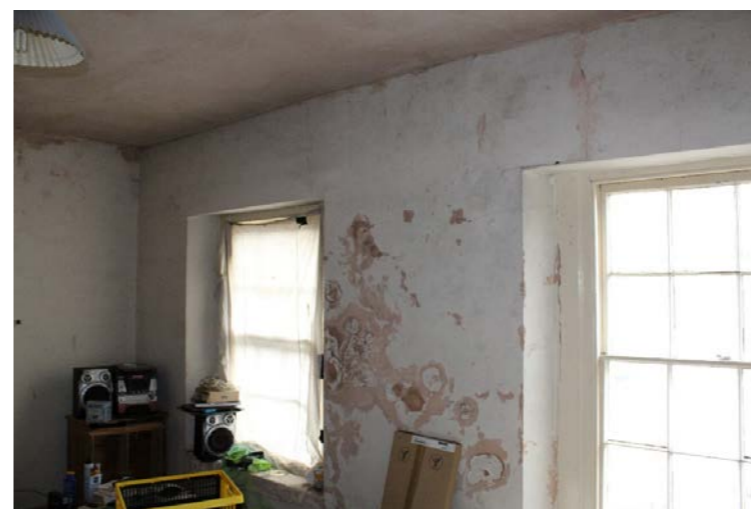
Fig. 8 Internal view of main building external walls - ingress of water has deteriorated wall/ceiling finishes and is in poor condition
