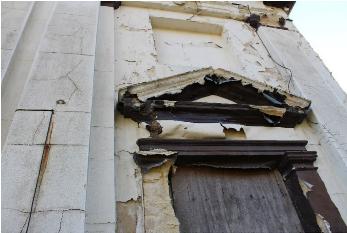
Fig.3 Inappropriate impervious render/paint applied to ornated external stonework has caused decay of the permeable stone below.
