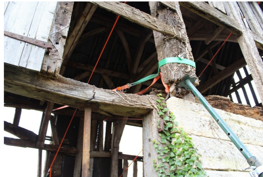
Fig.6 Temporary propping of frame preventing collapse where wall plate has rotted away.
