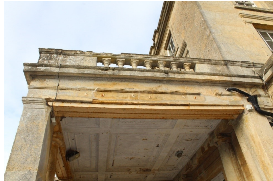
Fig. 4 Front porch - corrosion of exposed steel beam supports
