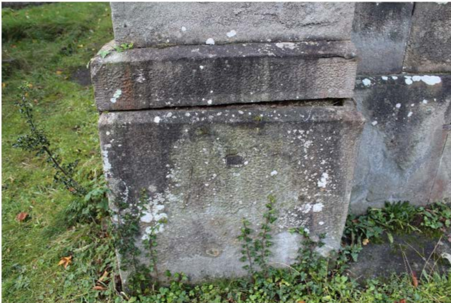
Fig.7 External stonework is defective
