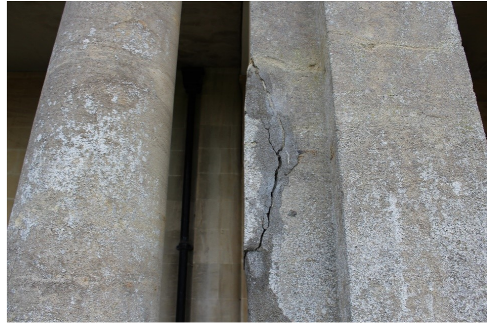
Fig. 14 Corrosion of steel work is cracking masonry walls
