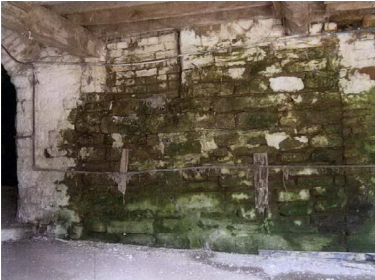
Damp internal walls (BEFORE)
