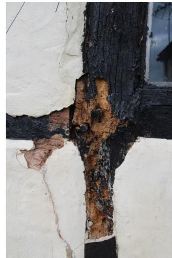
Fig 6. Trapped moisture is causing harmful decay of the original external timber frame
