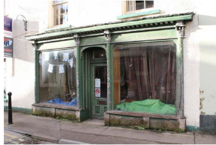
Fig. 2 Timber shop front - in poor condition
