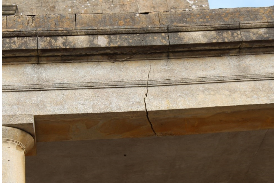
Fig. 5 Front colonnade - cracking evident in stonework
