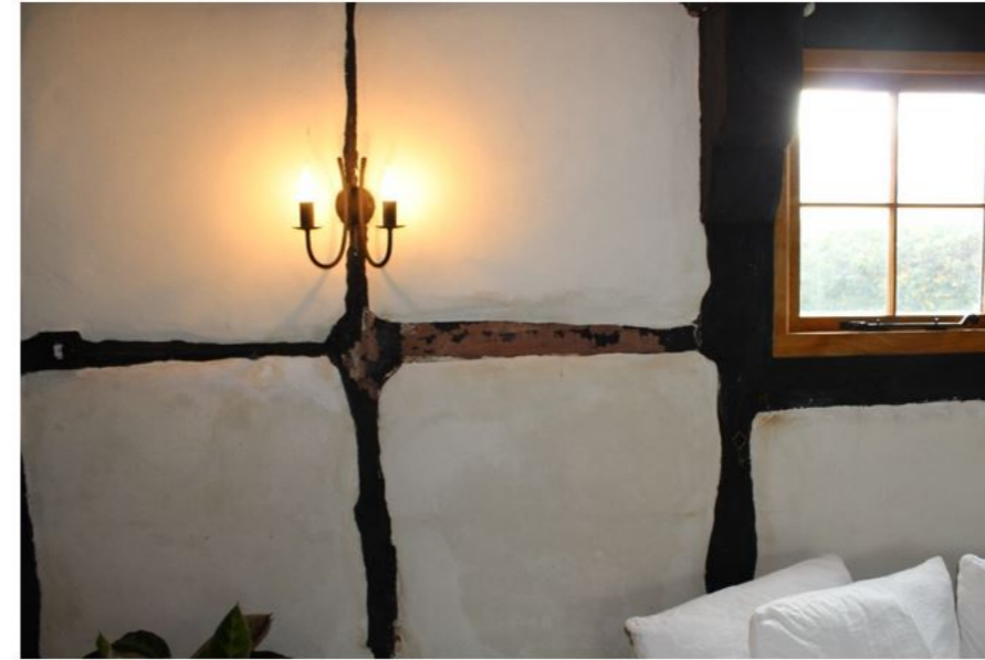
Fig.8 Trapped moisture is causing harmful decay of the original internal timber frame
