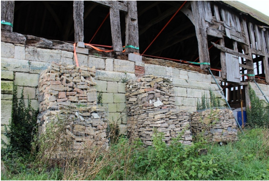
Fig.7 Gabion baskets provide temporary buttressing to prevent further movement and collapse of the outer walls.
