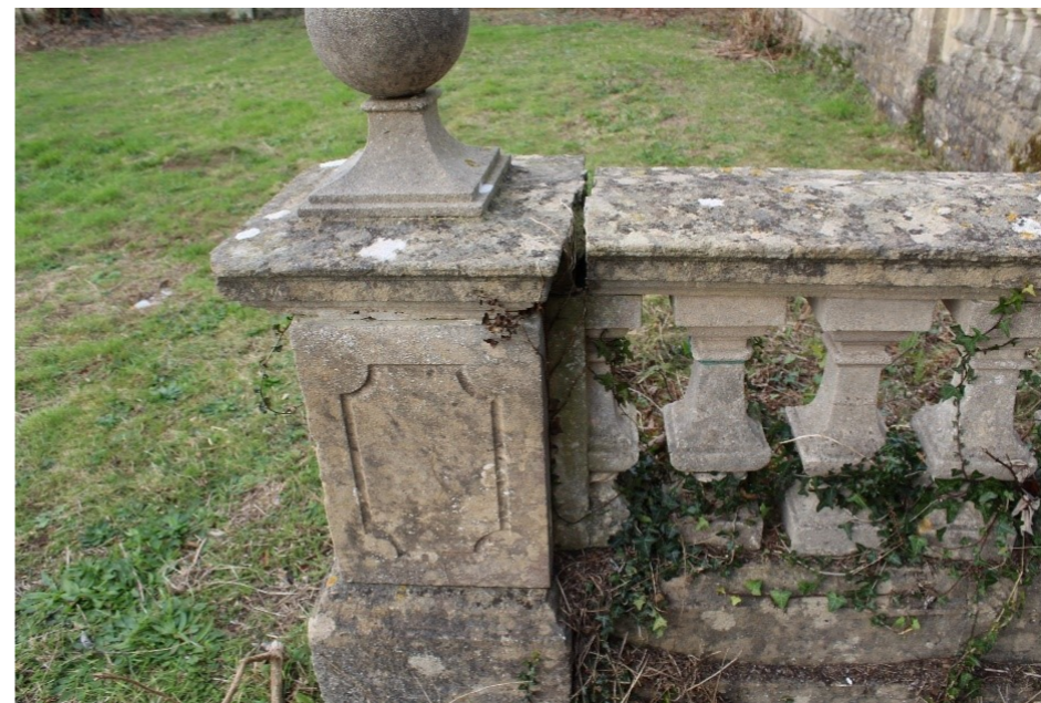
Fig. 18 Cracking evident in stonework
