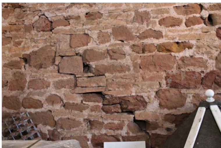
Fig. 7 Internal view of cracking evident in stonework
