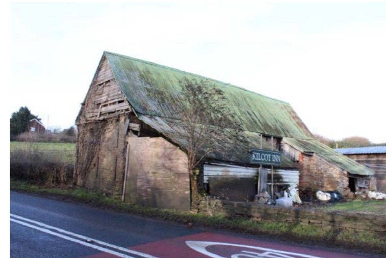
Fig. 2 Front and side elevation - in poor condition
