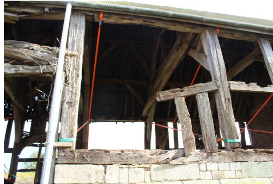
Fig.8 Timber frame exposed to the elements is severely deteriorated and collapsing from the building.
