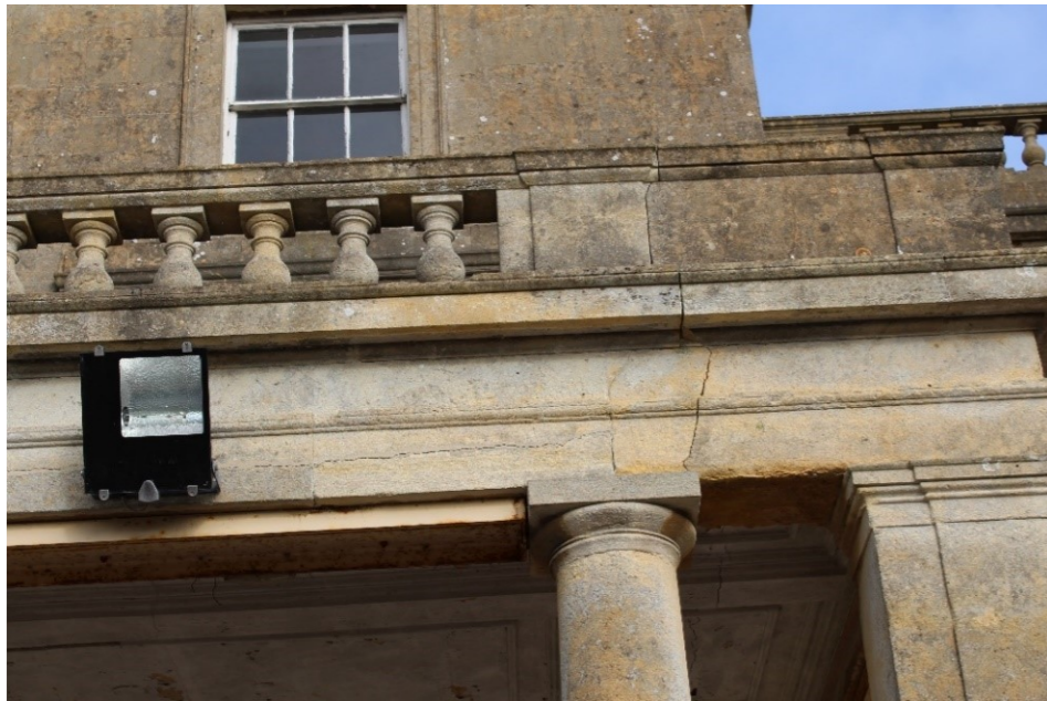
Fig.3 Front porch - cracking evident in stonework
