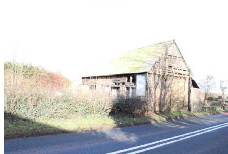
Fig. 4 Rear and side elevation - in poor condition
