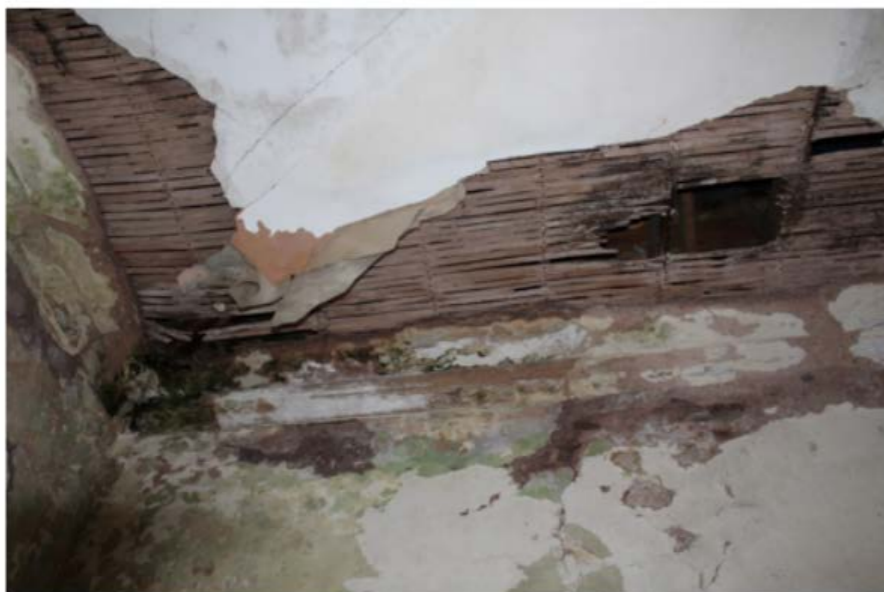
Fig. 13 Ingress of water has caused partial collapse of main ceiling finishes
