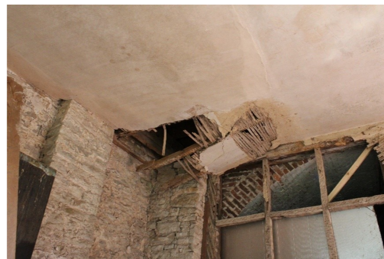
Fig. 6 Internal view of defective lath and plaster ceiling
