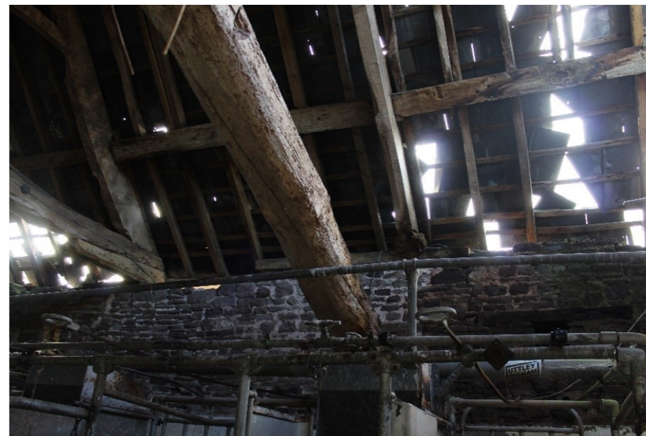
Fig.13 Internal View - Collapsed Tie Beam of Roof Truss
