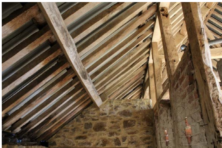
Fig. 6 Internal photo of barn viewed through a narrow wall opening - roof and walls structures appear in a stable condition
