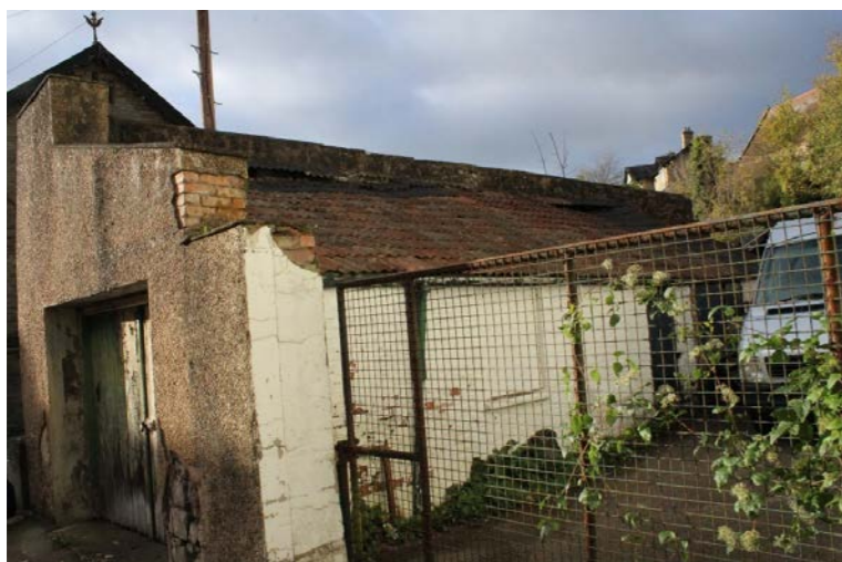
Fig. 5 Front and side elevation of detached curtilage listed garage - is in poor condition and roof has partially collapsed
