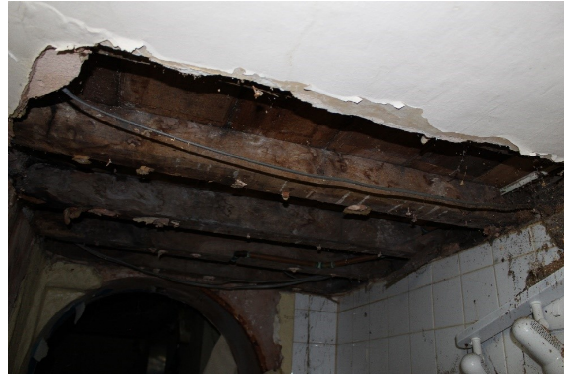
Fig. 4 Roof leaks have caused decay, collapsed and loss of the historic structure below in multiple areas over 3 floors.
