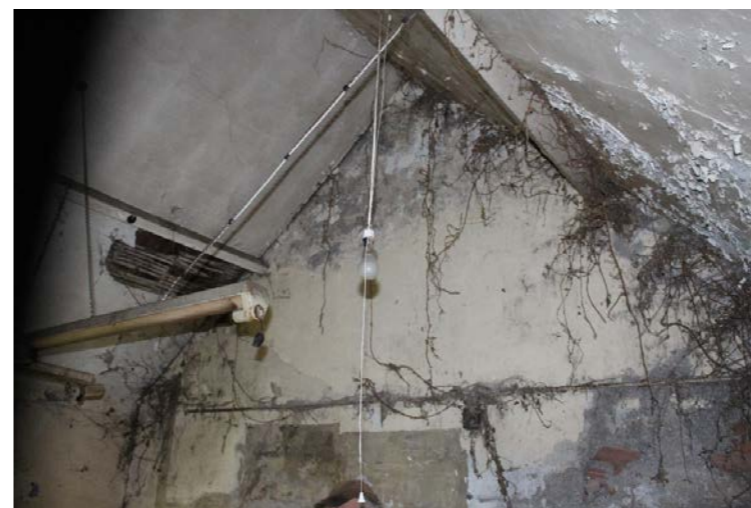
Fig. 10 Internal view of print works building - ingress of water has deteriorated finishes; the ceiling and timber floor has partially collapsed and is in poor condition
