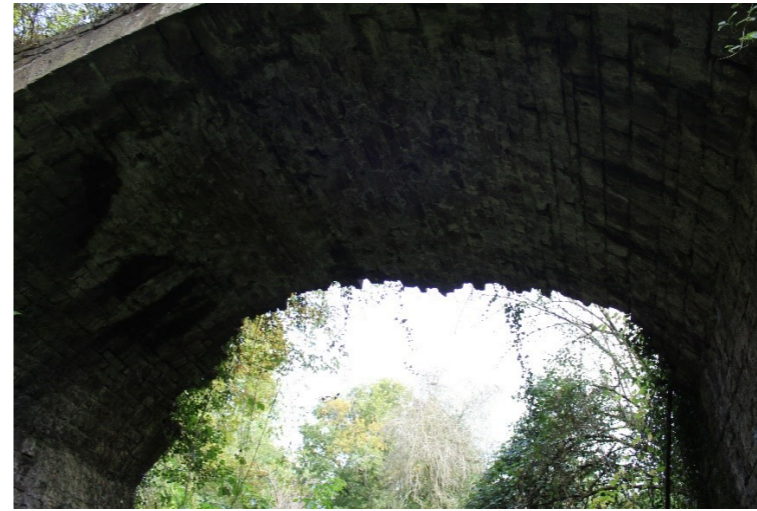
Fig. 6 Intrados of central arch with face voussoirs missing on upper road side
