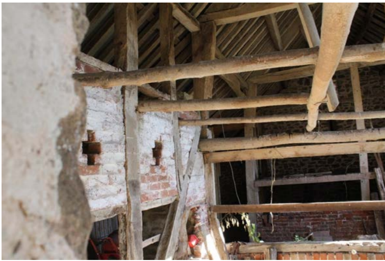
Fig. 4 Internal photo of barn viewed through a narrow wall opening - roof and wall structures appear in a stable condition
