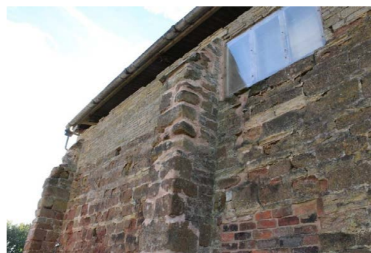
Fig. 10 Modern repointing of buttress
