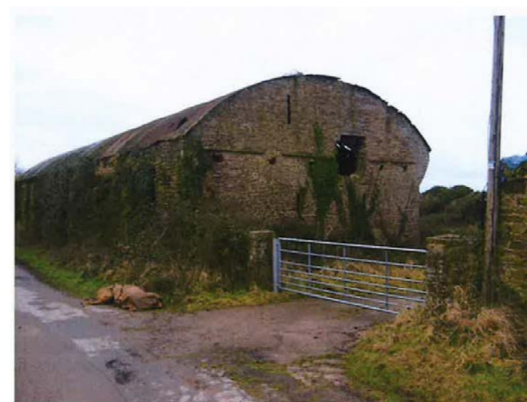
Main barn dilapidated 2009
