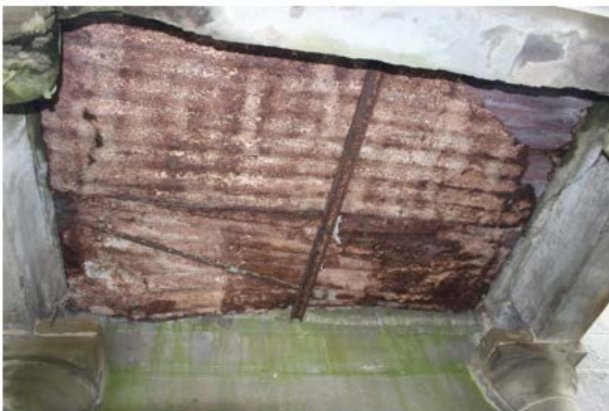
Fig. 9 Front porch roof soffit is deteriorating
