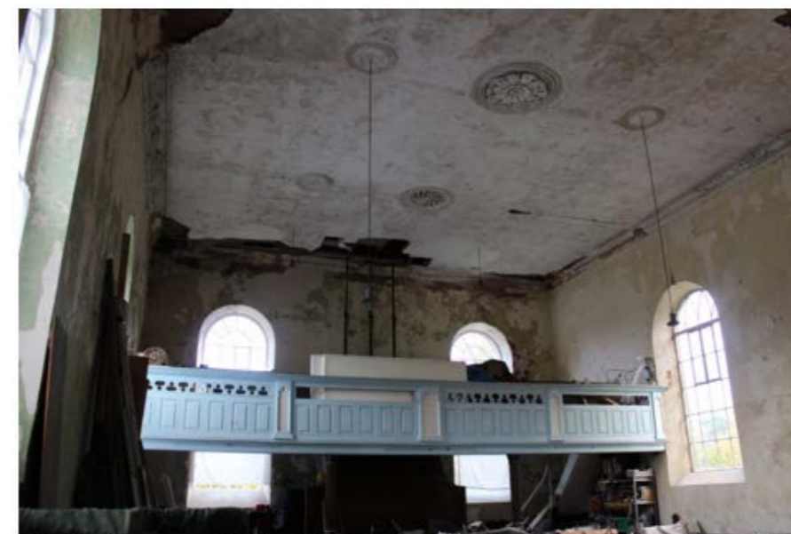
Fig. 12 Ingress of water has caused partial collapse of main ceiling finishes
