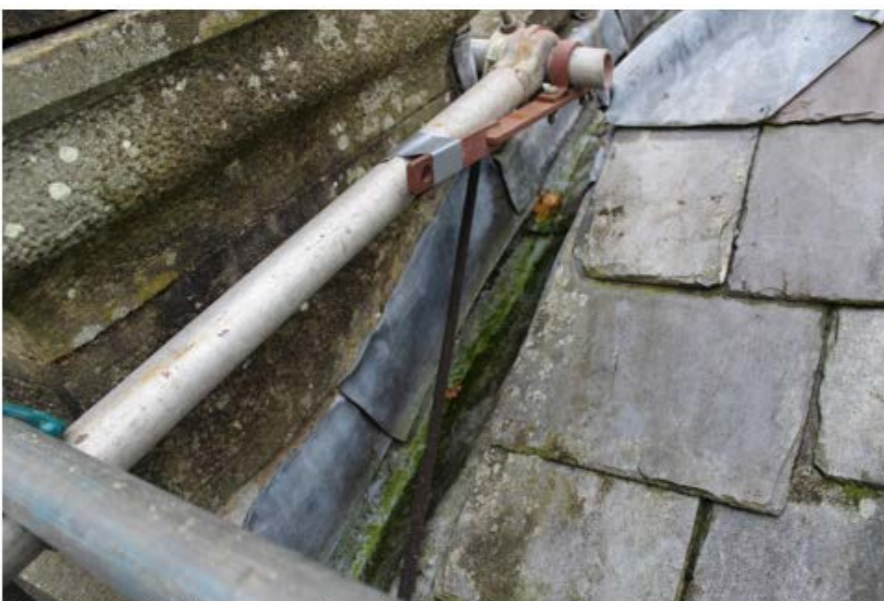
Fig.11 Defective parapet gutter is allowing ingress of water into the building
