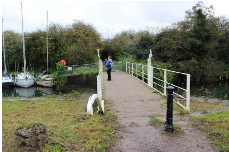
Fig.3 Swing Bridge requires repairs to operate again.
