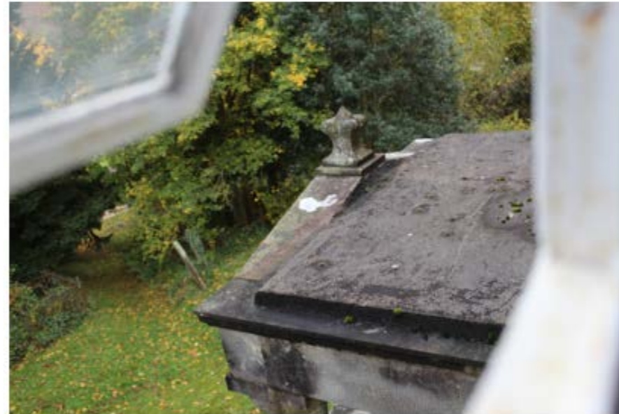
Fig.8 Front porch roof has no weather protection
