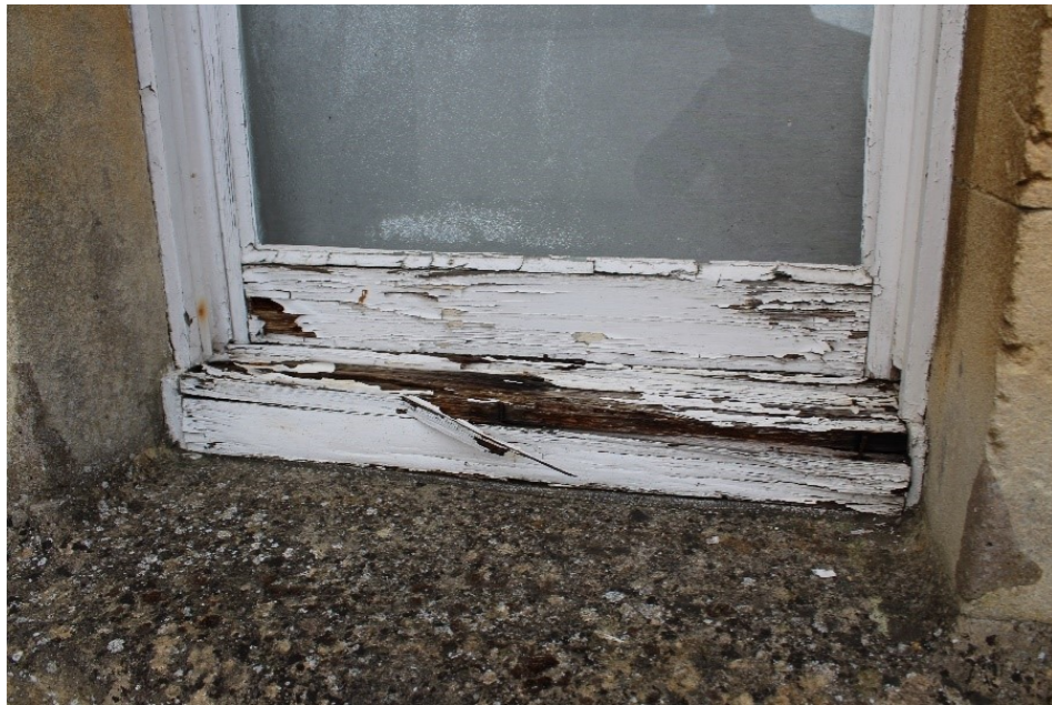
Fig. 11 Defective timber windows
