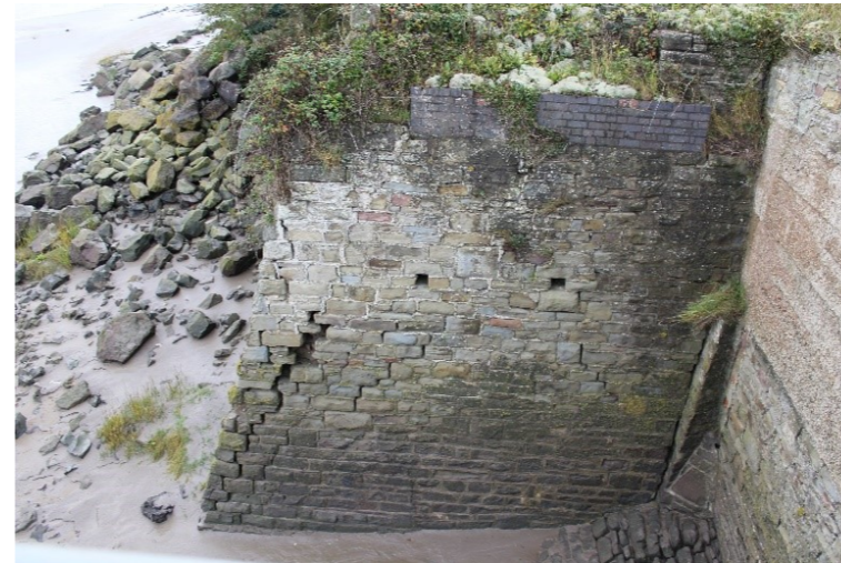
Fig.4 Defective stonework to sluice outfall requires repair.
