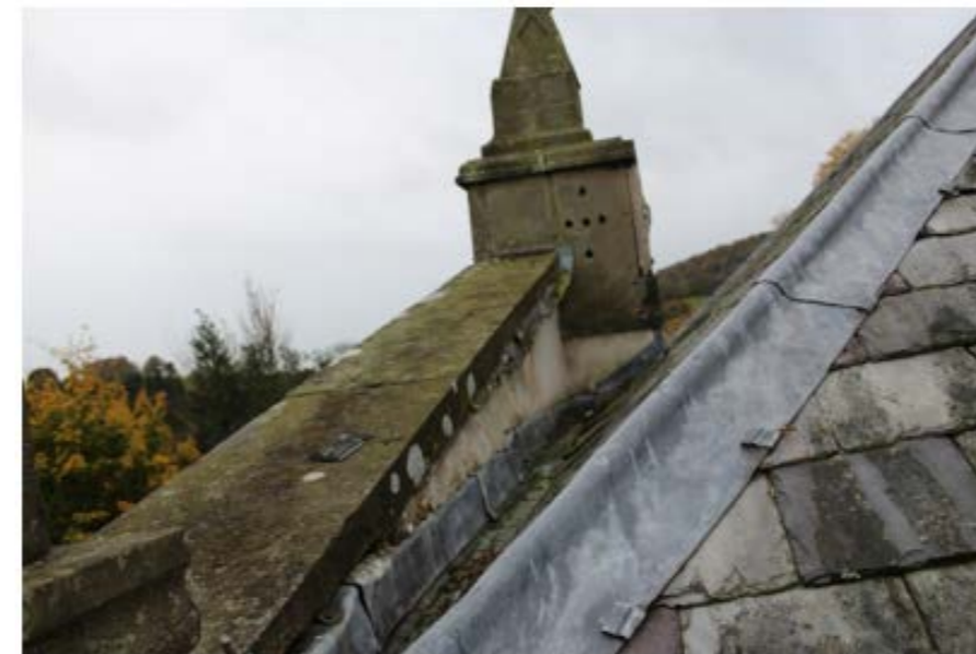
Fig. 10 Defective parapet gutter
