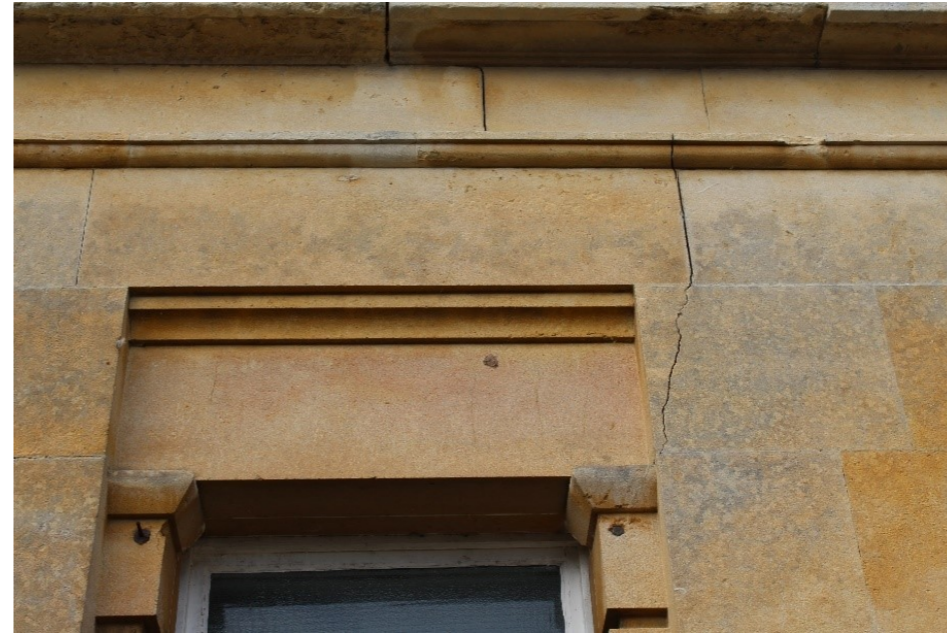
Fig. 10 Rear elevation - cracking evident in stonework
