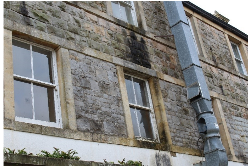
Fig. 12 Defective timber windows
