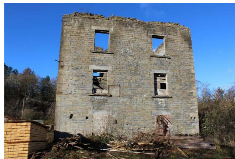
Fig.2 Side elevation - original lean too was up to underside of first floor stone sills
