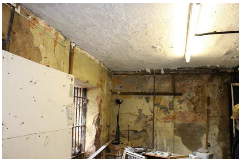
Fig. 9 Internal view of rear building - ingress of water has deteriorated wall/ceiling finishes and is in poor condition
