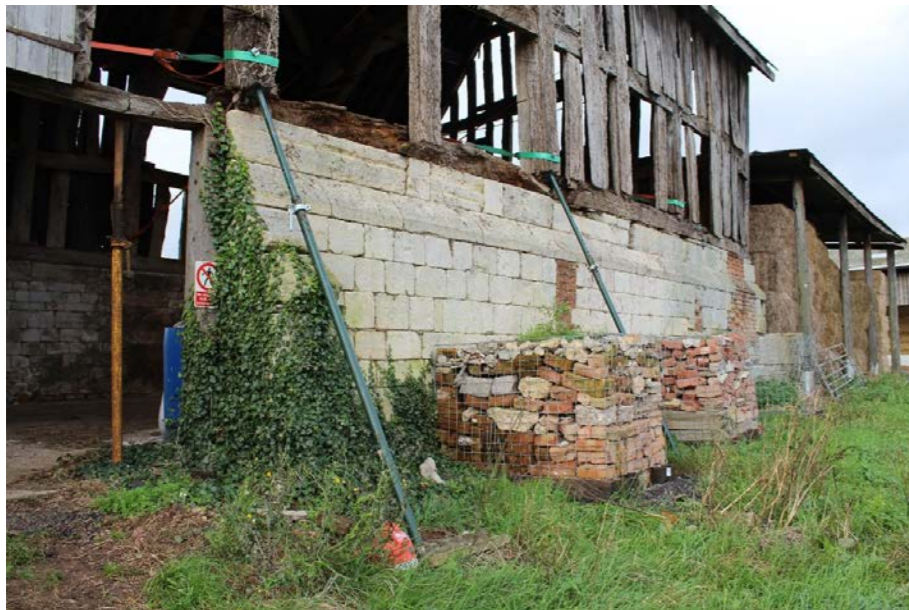
Fig.5 Temporary propping of frame preventing collapse where wall plate has rotted away.
