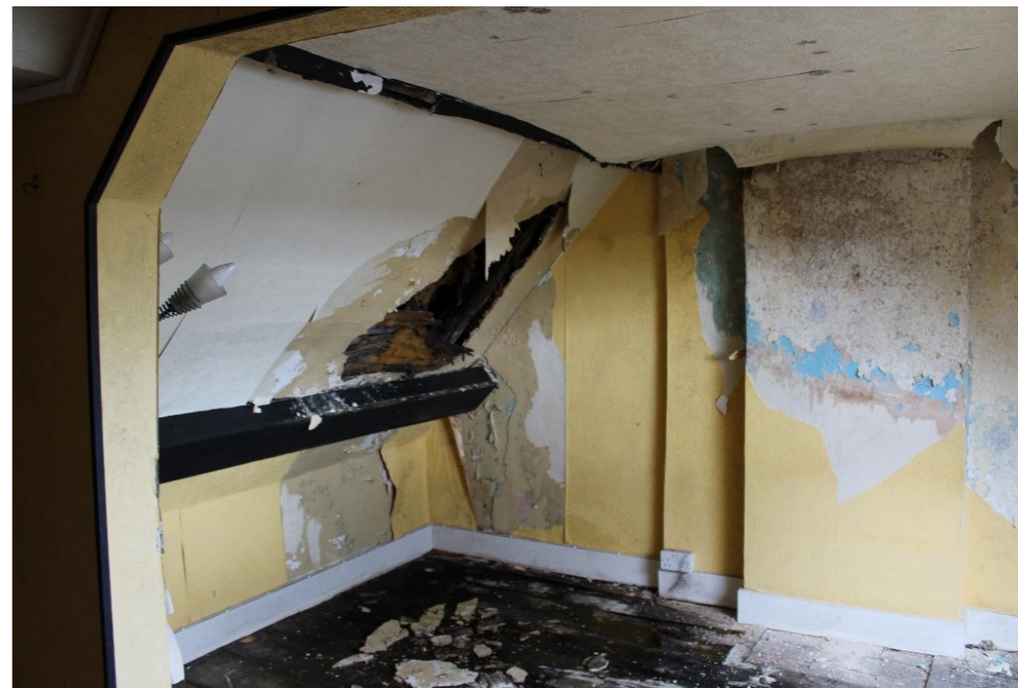
Fig. 10 Roof leaks have caused decay, collapsed and loss of the historic structure below in multiple areas over 3 floors.
