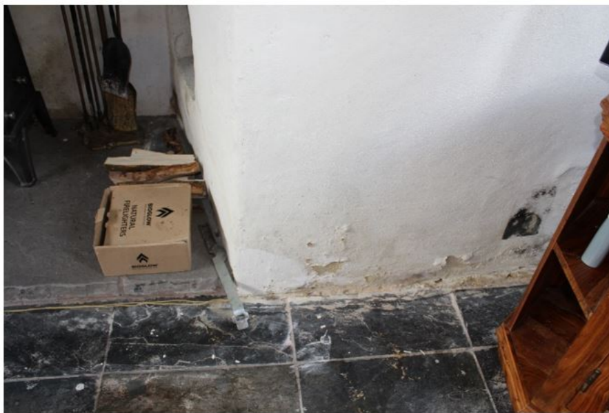
Fig.9 Modern hard impervious plasters and paints applied to internal walls are trapping moisture and causing decay
