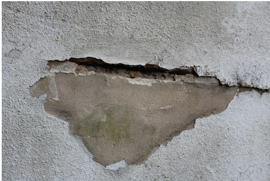
Fig. 15 Corrosion of steel work is cracking masonry walls
