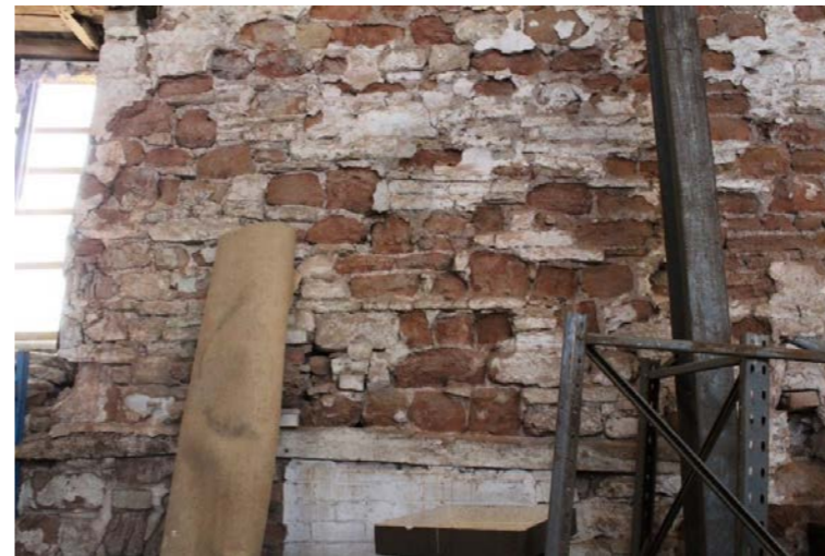
Fig. 6 Internal view of decaying stonework and defective lime pointing
