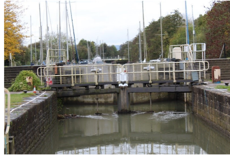
Fig.2 Lock gate and tidal exclusion gate require repair.
