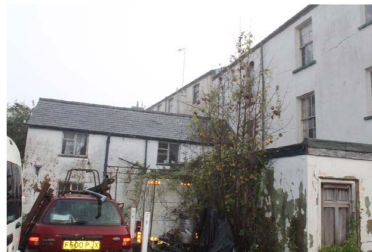
Fig. 6 Rear elevation - deep cracking is evident in external walls and is generally in poor condition
