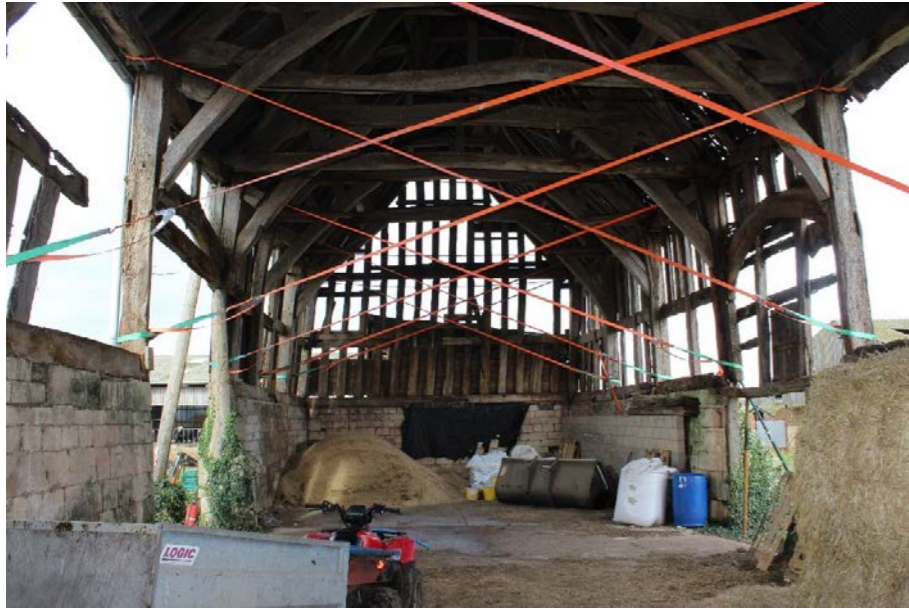
Fig.3 Temporary strapping restraining frame and preventing collapse. Stored materials still accessed by heavy farm machinery.
