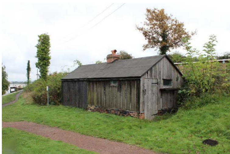
Fig.7 Generator shed and wages office requires repair.
