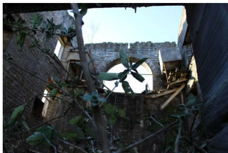
Fig. 5 Internal view with water tanks visible at high level - access was restricted
