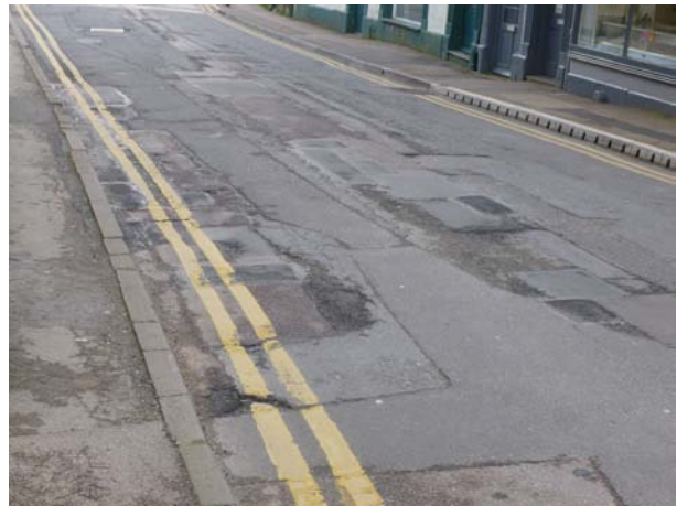
Figure 95 - Poor road surfaces on Newland Street
