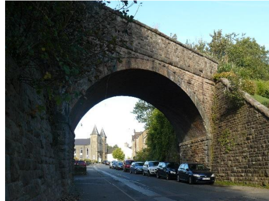
H13 Viaduct is a prominent feature, leading toward the FODDC offices from the Angus Buchanan.
