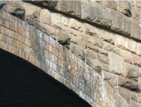
H12 The viaduct is red forest dressed sand stone, with Coleford bricks around the arch. Also known as the Skewed Bridge because of its shape.
