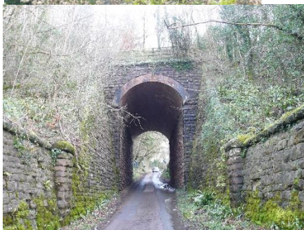
12. The dressed red Forest stone is used for the retaining walls and Whitecliff bridge, but Coleford bricks form the arch and this is carried right underneath.
