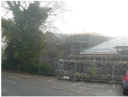
D6 Parkside overlooks this new extra care development here under construction on the old Community Centre site off Bank St.
