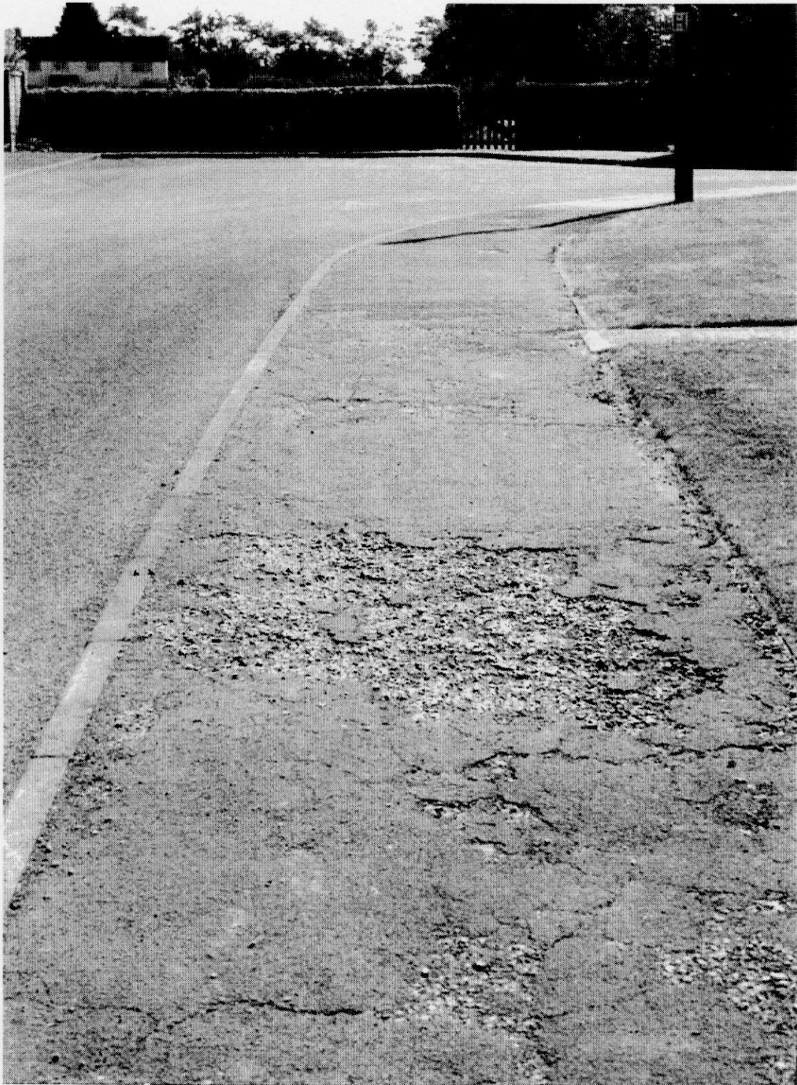
Worn out pavements in Westwick Road
