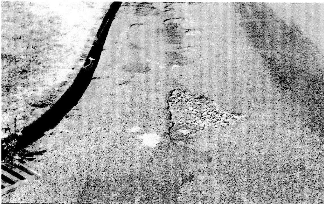
Worn out road surface in Sunset Place.
