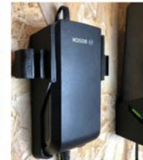
Wall mounted electric charging
