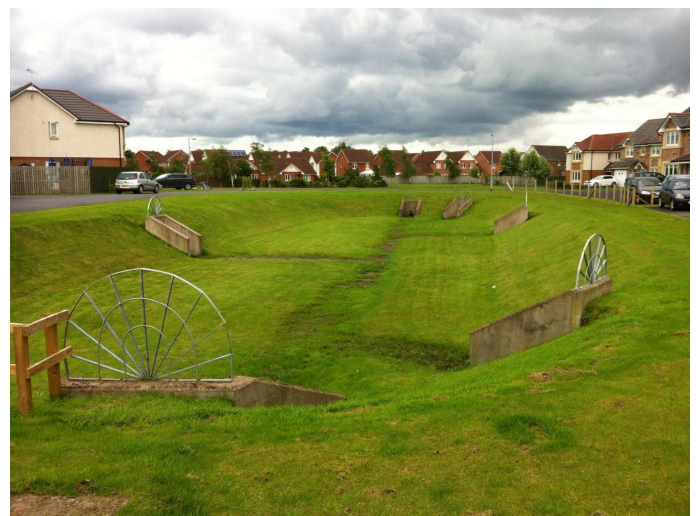
Figure 10-10 – Poor headwall design
