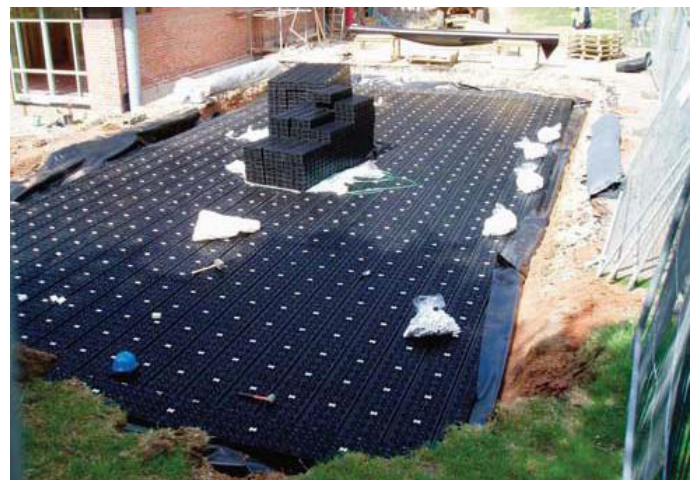
Figure 9-45 – Geocellular boxes used as sub-base for permeable pavement
