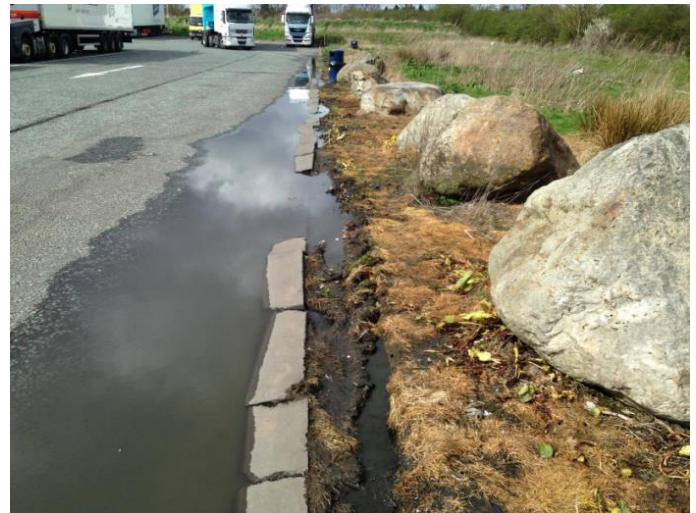
Figure 9-12 – Filter strip showing need of maintenance
