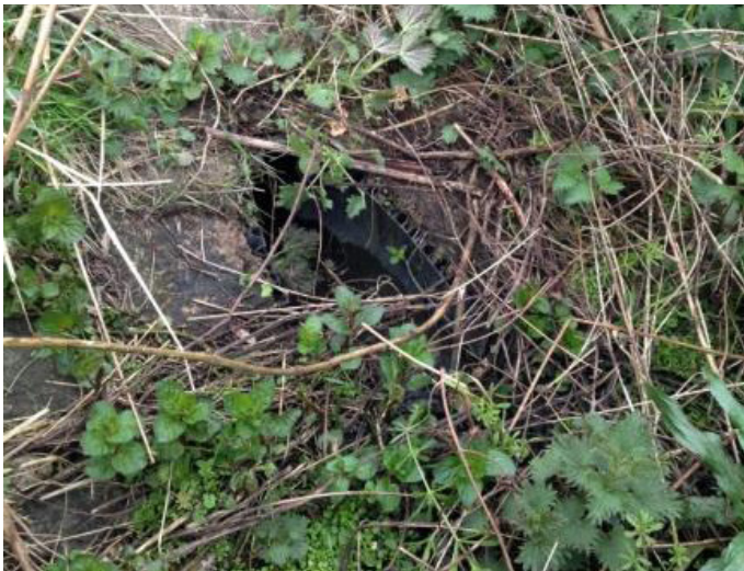
Figure 10-11 – Pipe inlet in need of maintenance
